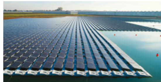
Mega-projects have helped to make SABIC one of the best climate change performers in the Middle East.
